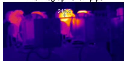
Thermograph of compressor system
