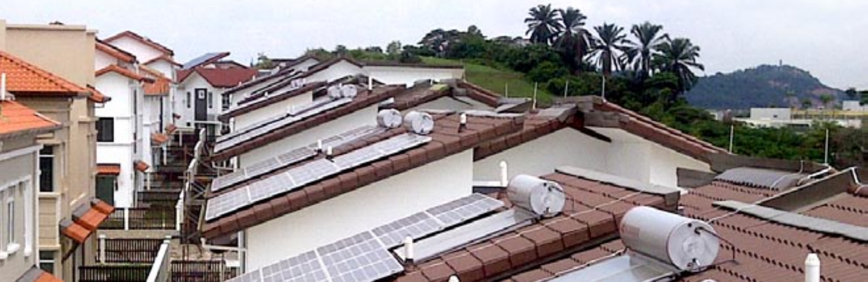
Kediaman di Setia Eco Park fasa 11A-34 (fotovolta suria dengan kapasiti 4 kW bagi setiap rumah) Residential units at Setia Eco Park Phase 11A-34 (houses with solar PV capacity of 4 kW each)
