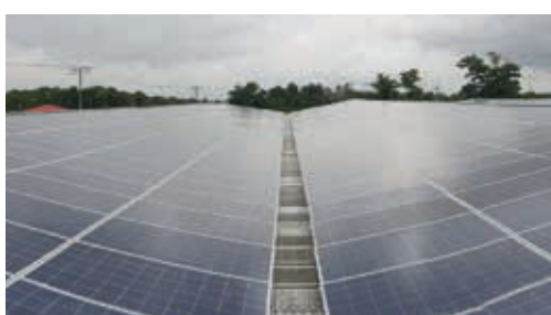
Solar Farm of Kuala Penyu, Sabah, 1700kWp
