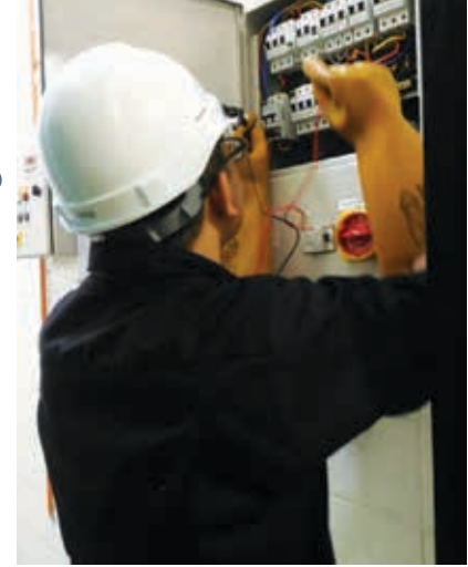
A technician inspecting an electrical circuit as part of the energy audit process.
