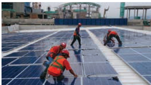
MITI Building, 100kWp
