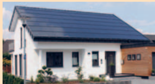
Roof integrated PV system with frameless CIGS tin film modules, courtesy of Wurth Solar /Germany
