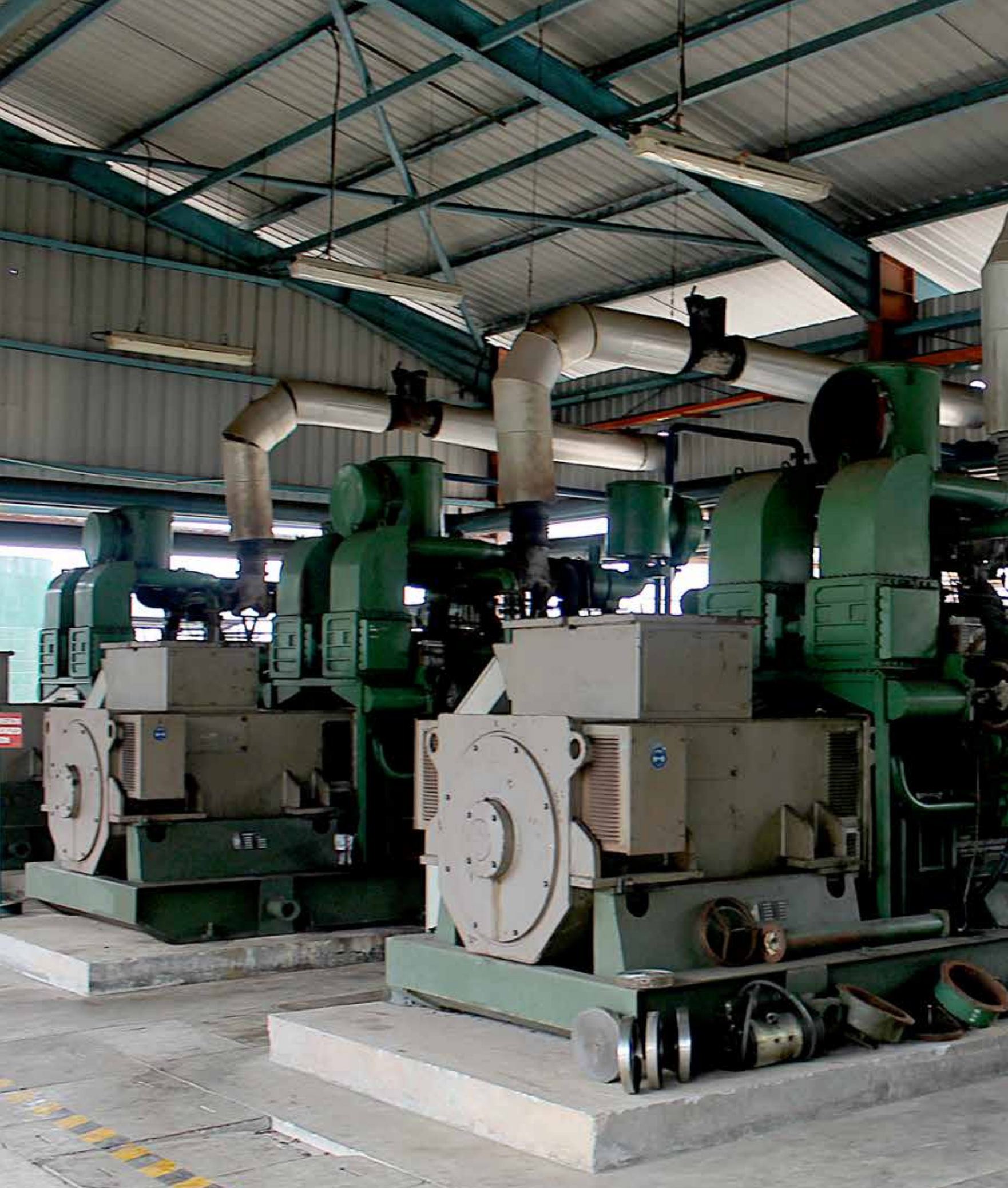
Janakuasa Biogas 2 MW, Bell Eco Power Sdn Bhd, Batu Pahat, Johor. / 2 MW Biogas Power Plant, Bell Eco Power Sdn Bhd, Batu Pahat, Johor.
